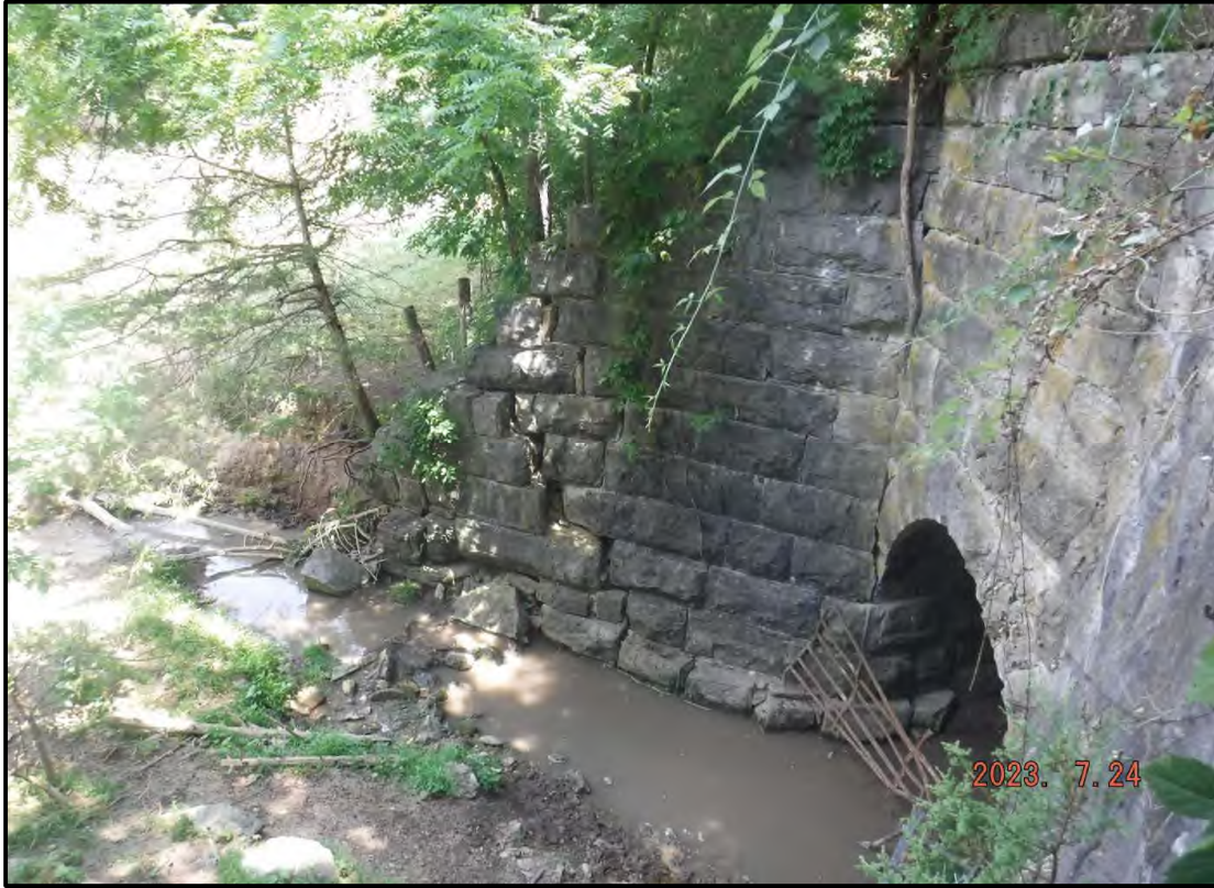
Photo 5: NE Wing with Free End Separation
