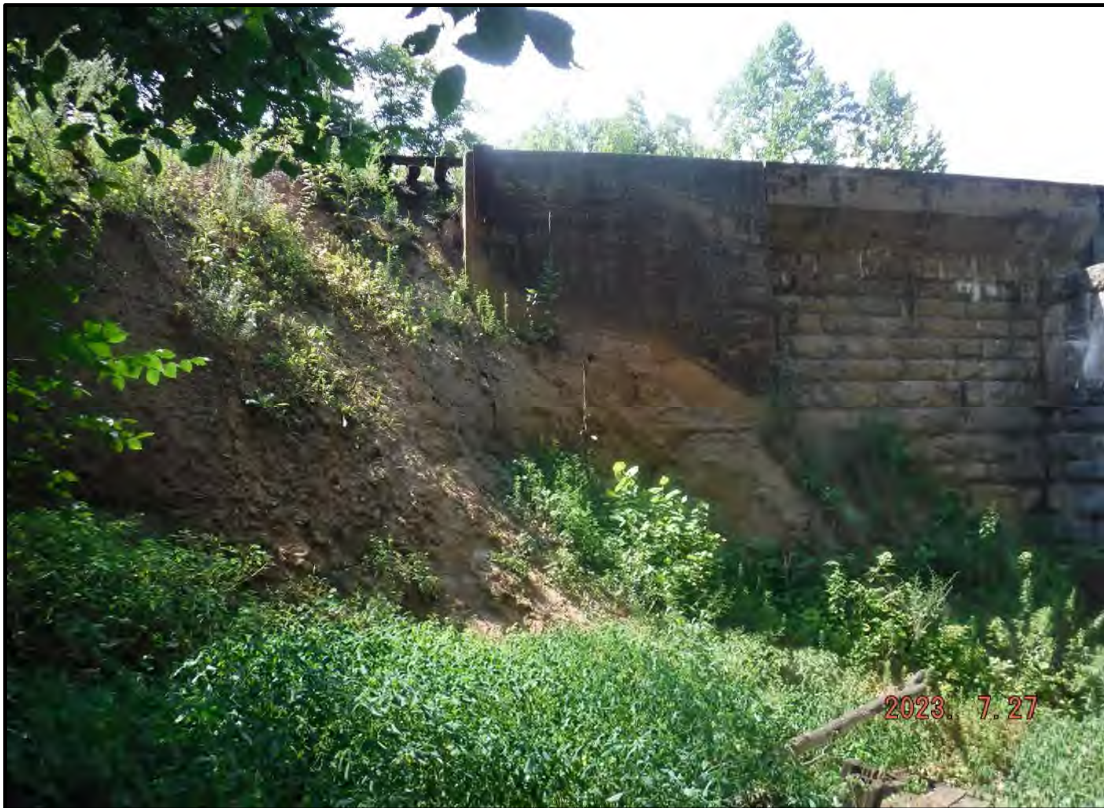
Photo 2: Erosion/Washout at SW Corner of Structure
