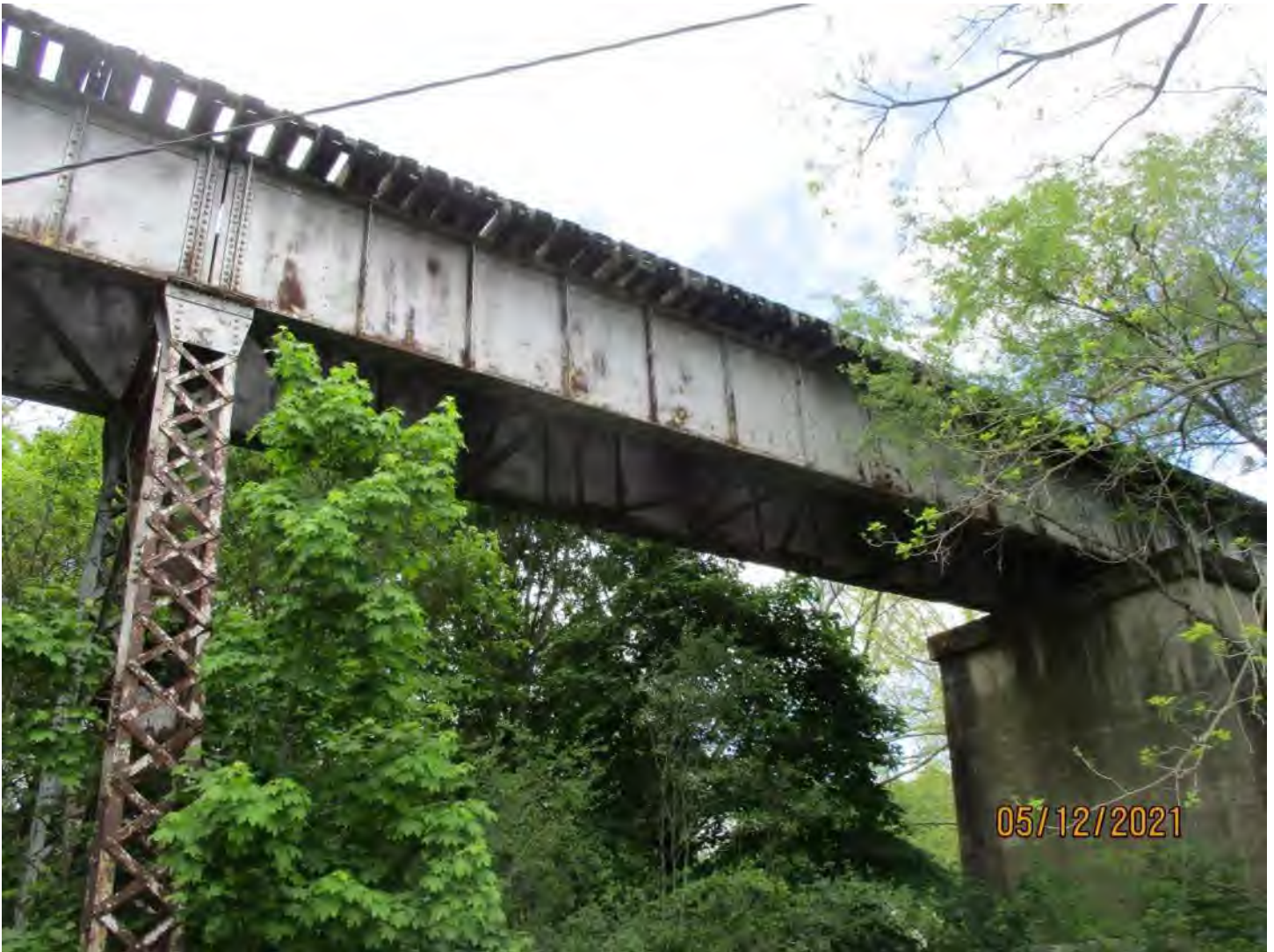
Asset 7902 over Stoney Creek and Massie Farm Lane N 38° 49' 22.27", W 78° 34' 10.06" Seven Span Steel Girder Bridge, 375'-0"
