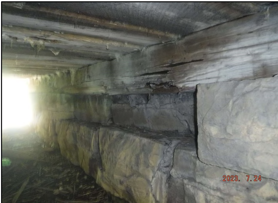
Photo 4: Spalled/Broken Stones At South End of West Abutment
