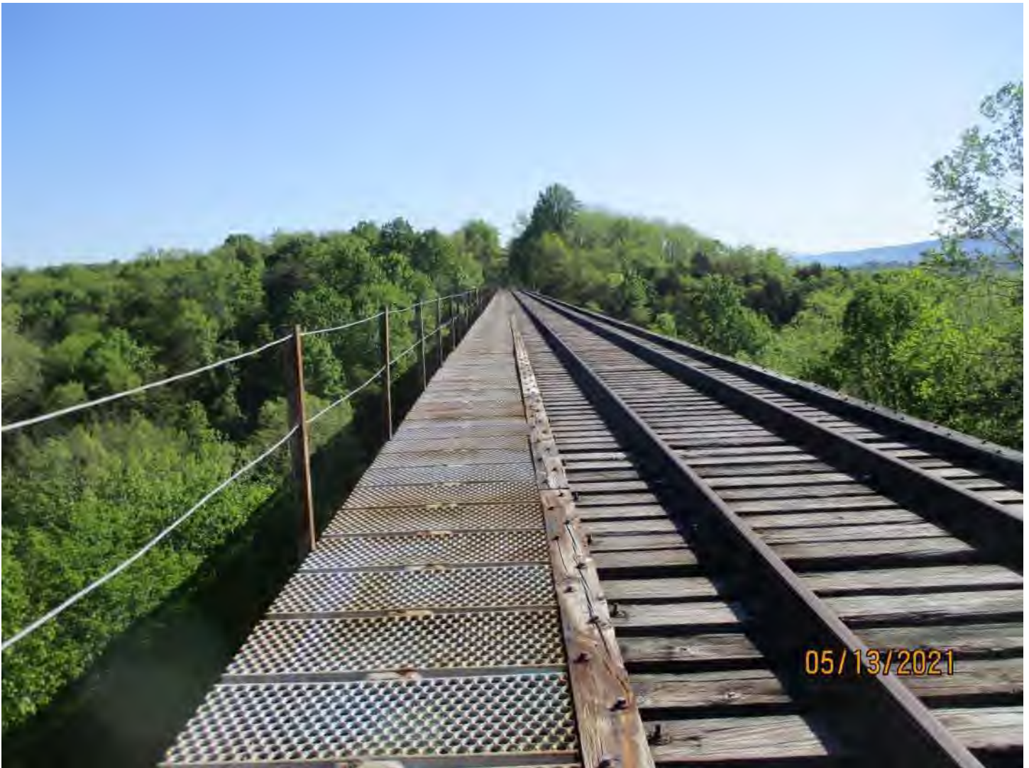
Asset 7643 over Narrow Passage Creek N 38° 50' 45.03", W 78° 32' 12.71" Seven Span Steel Girder Bridge, 630'-0"
