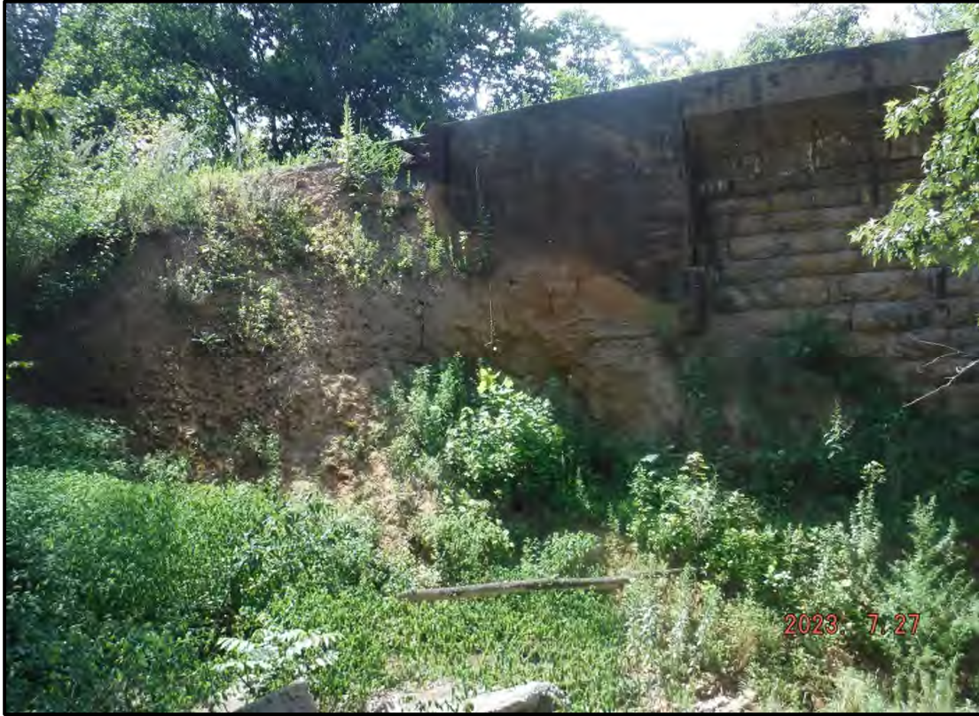
Photo 1: Erosion/Washout at SW Corner of Structure
