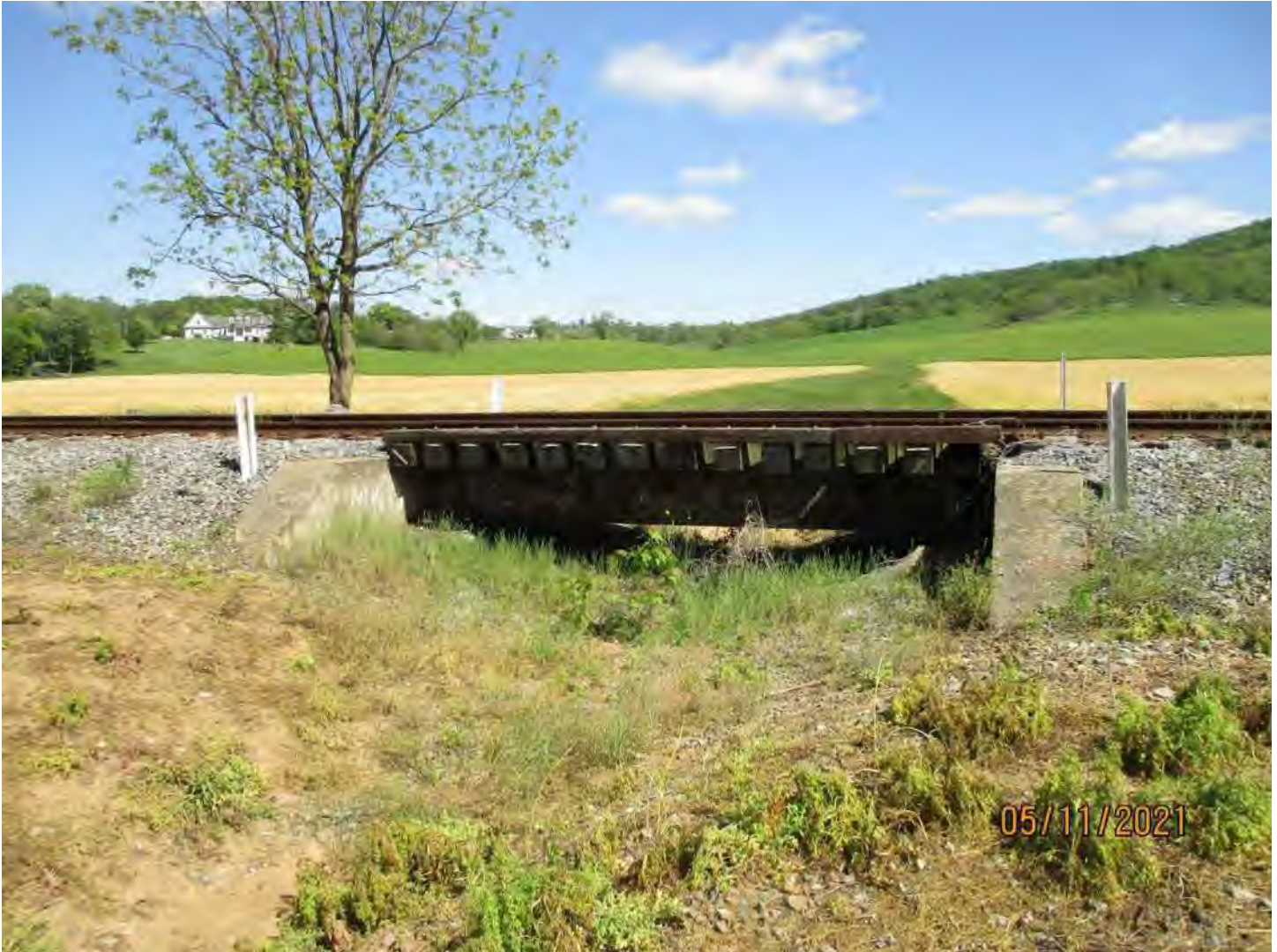
Asset 9571 over Unnamed Drainage Crossing N 38° 38' 45.65", W 78° 44' 54.96" Single Span Steel Girder Bridge, 19'-8"
