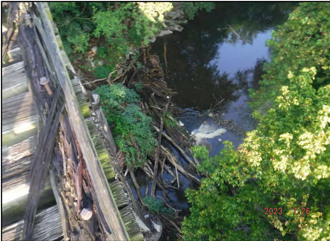
Photo 2: Flood Debris Against the North Side of the Steel Bent Tower
