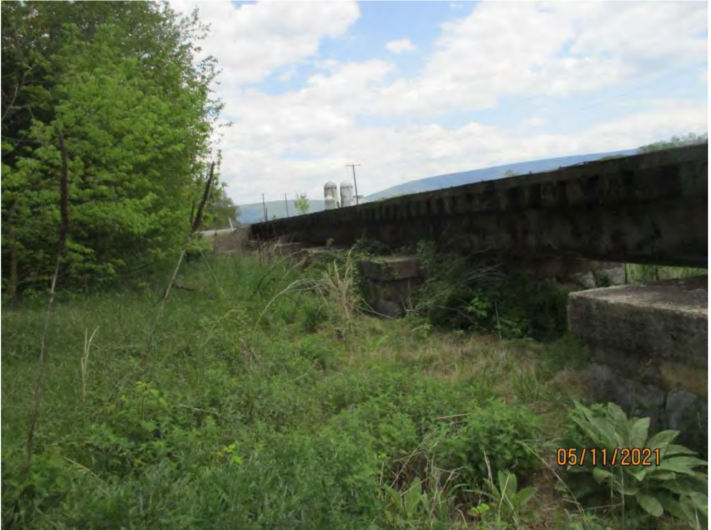
Asset 9430 over Unnamed Drainage Crossing N 38° 38' 58.39", W 78° 43' 22.10" Seven Span Steel Double Girder Unit Bridge, 140'-4"
