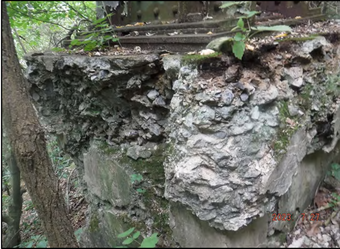
Photo 7: Spalled Concrete on Main Span Bent 2 North Pedestal
