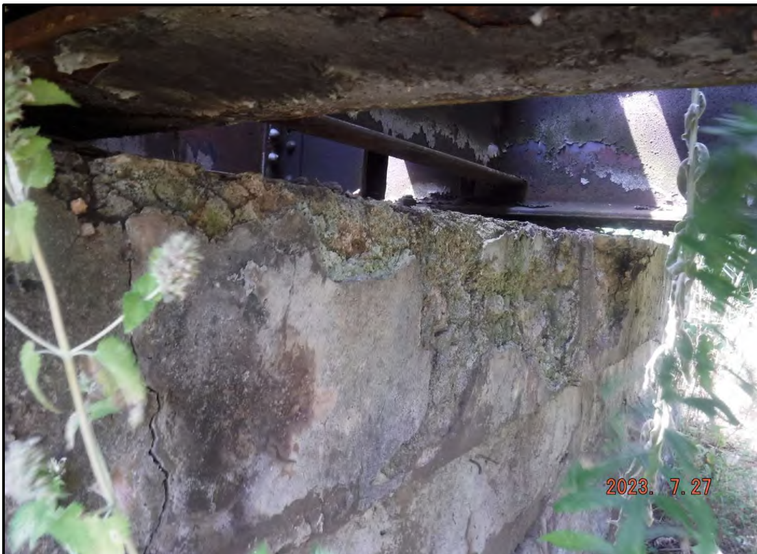
Photo 6: Typical Spalled Bridge Seat (Outside of Bearings)
