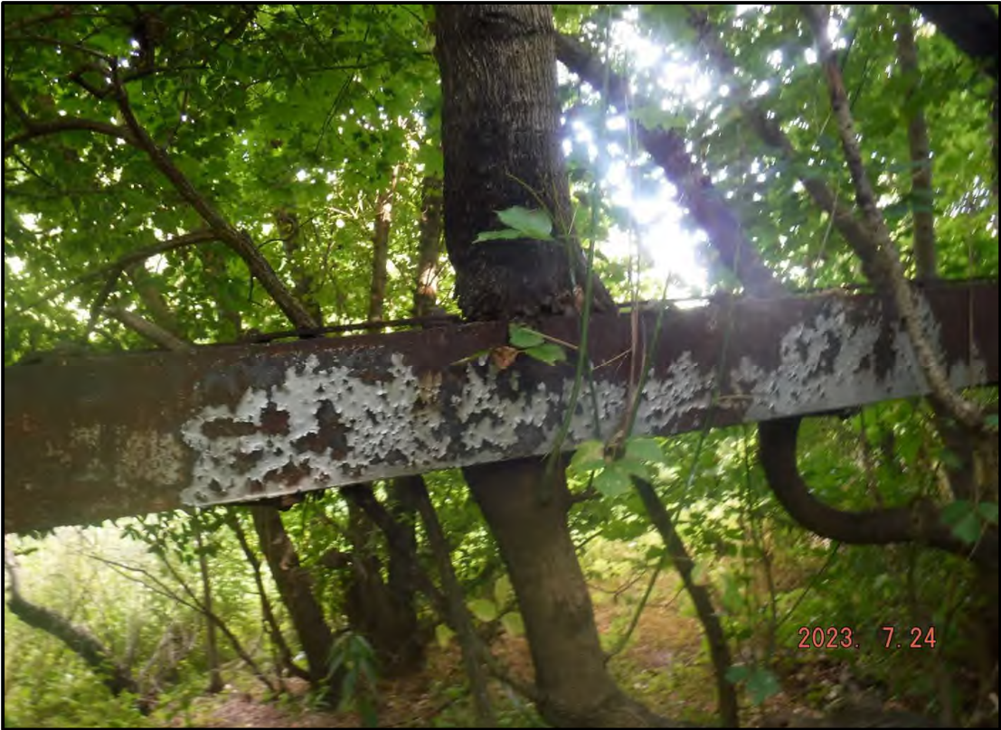
Photo 2: Vegetation Growth in Steel Bent Tower Bracing
