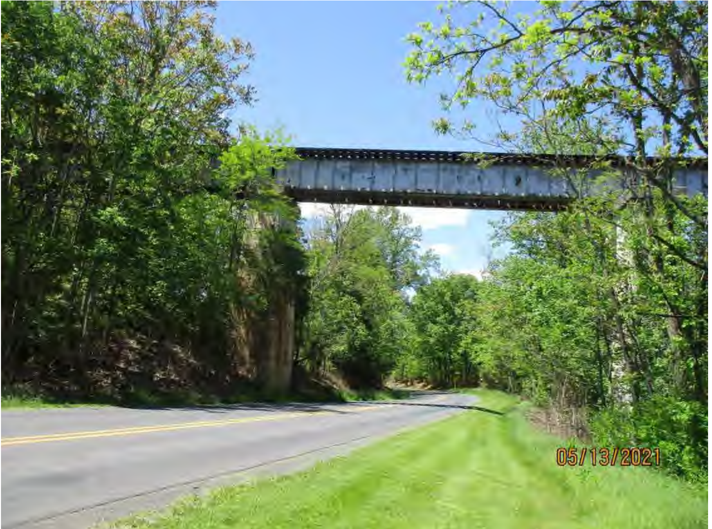
Asset 6391 over Battlefield Rd and Tumbling Run N 38° 59' 3.73", W 78° 23' 50.09" Four Span Steel Two Girder Bridge, 262'-0"
