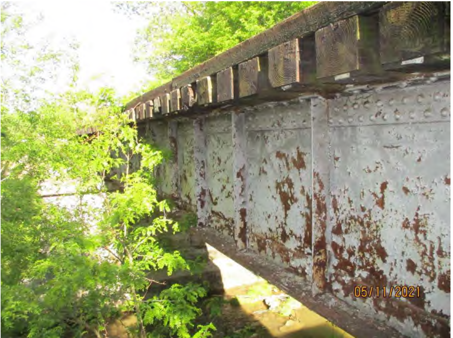
Asset 9736 over Honey Run Creek N 38° 38' 20.06", W 78° 46' 33.80" Two Span Steel Girder Bridge, 90'-0"
