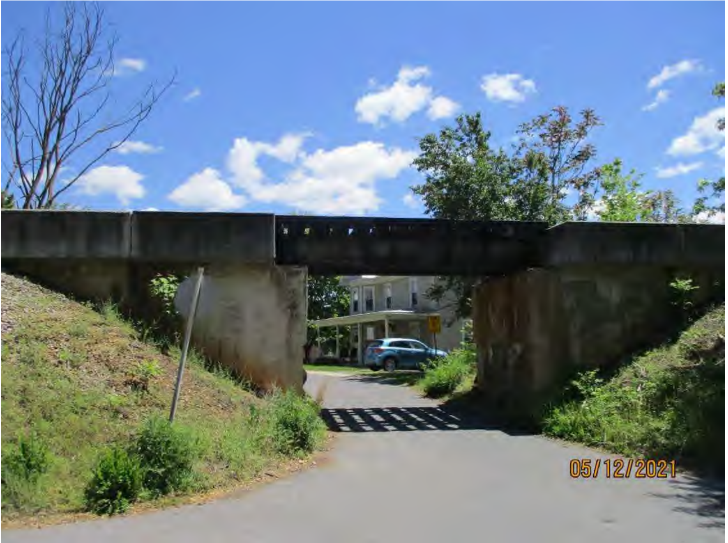
Asset 8620 over Bank Street N 38° 44' 40.55", W 78° 38' 42.92" Single Span Steel Double Girder Unit Bridge, 20'-10"
