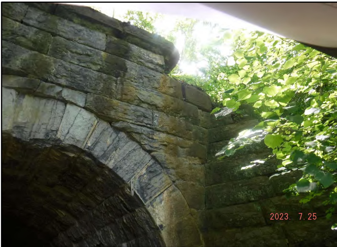
Photo 2: Missing Stones West End of North Headwall
