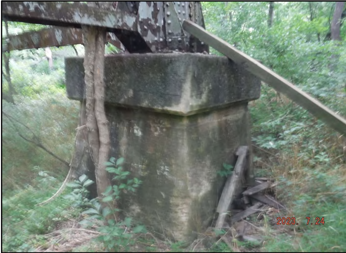
Photo 4: Typical Steel Bent Tower Pedestal
