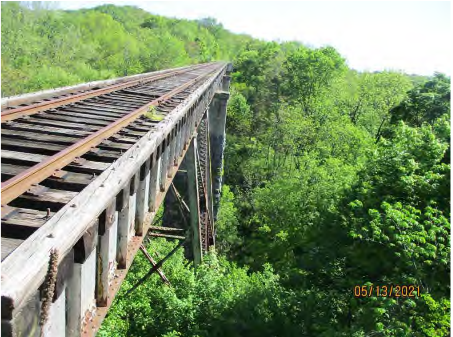
Asset 7164 over Pughs Run N 38° 54' 12.88", W 78° 29' 24.81" Nine Span Steel Two Girder Bridge, 380'-0"
