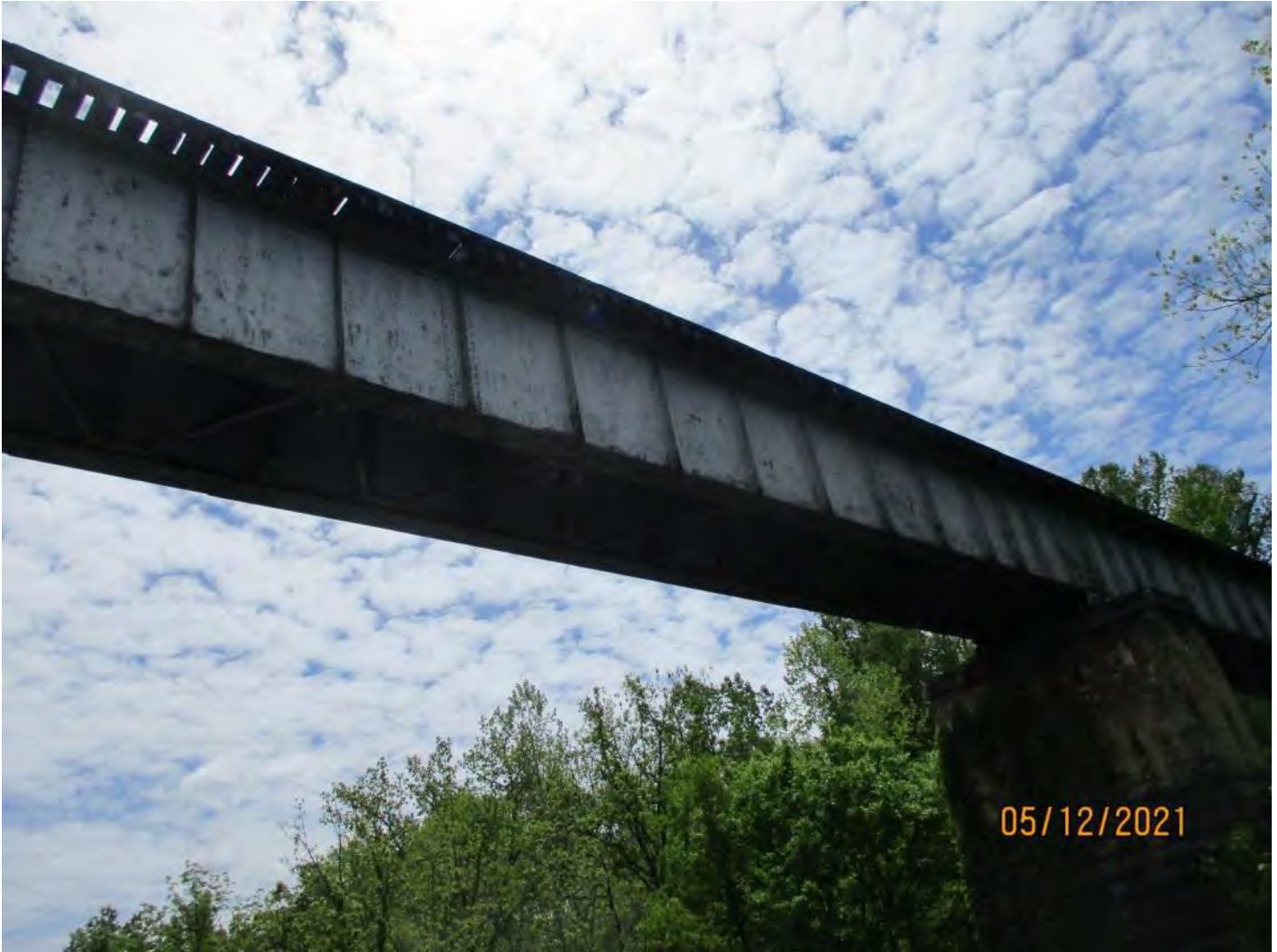
Asset 8627 over North Fork Shenandoah River and Bryce Blvd N 38° 44' 37.22", W 78° 38' 45.09" Three Span Steel Girder Bridge, 425'-0"
