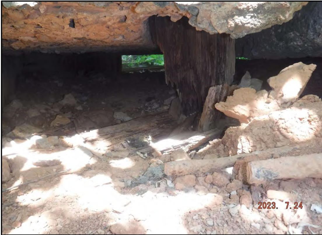
Photo 5: Undermined East Approach Ballast Trough
