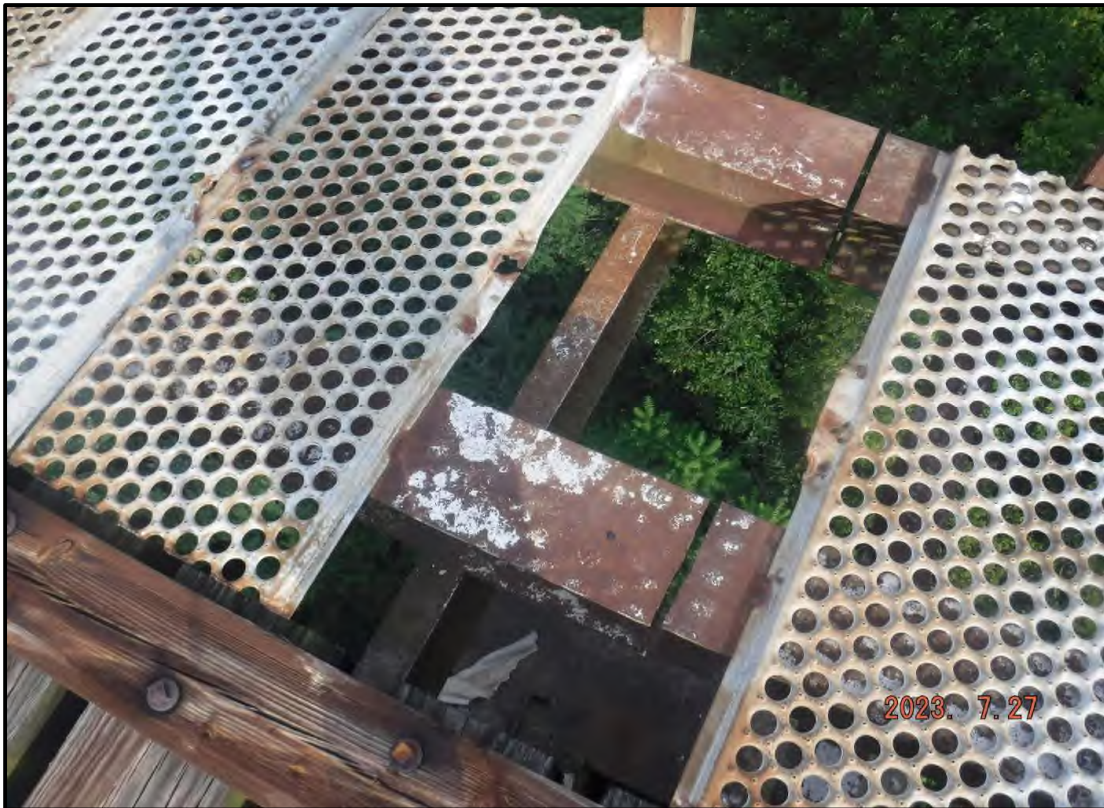
Photo 2: Missing Walkway Grate over Pier 3 of Main Spans
