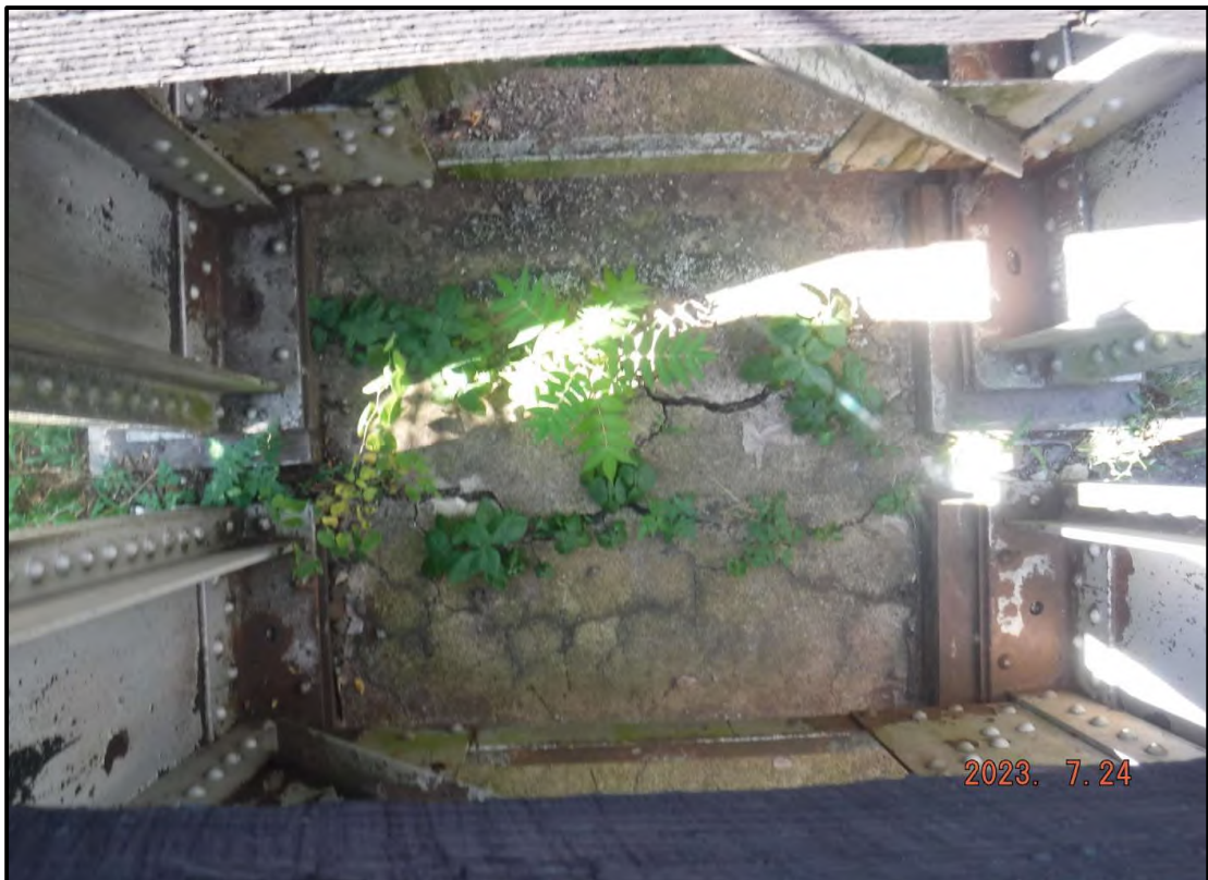
Photo 2: Pier 3 Bridge Seat With Wide Cracks
