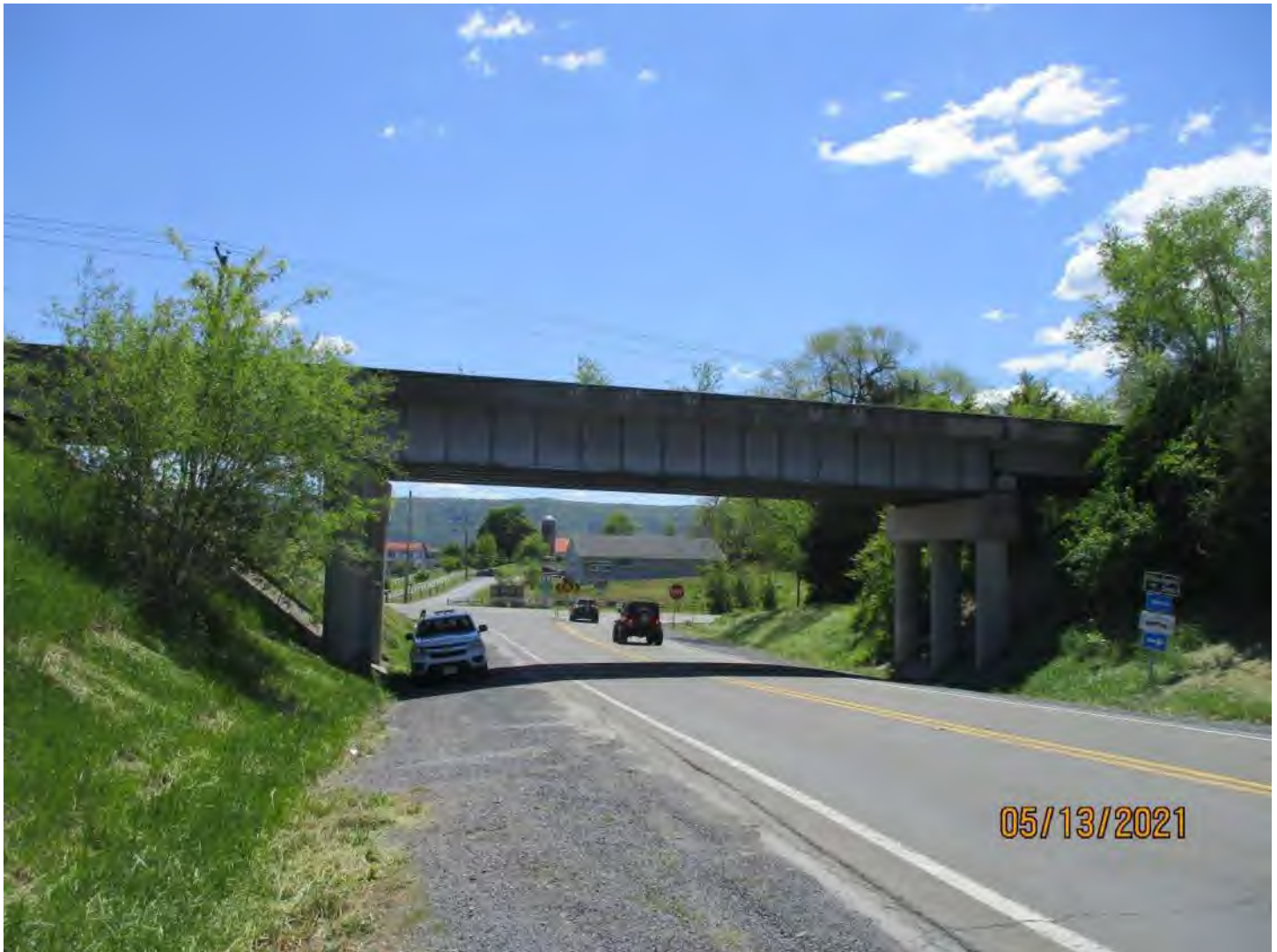
Asset 6669 over Rte 651 Mt Olive Rd N 38° 57' 17.50", W 78° 25' 43.73" Three Span Steel Girder Bridge, 127'-0"
