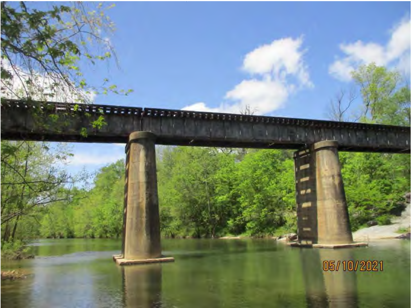
Asset 9970 over North Fork Shenandoah River N 38° 38' 11.38", W 78° 46' 51.59" Four Span Steel Girder Bridge, 184'-0"
