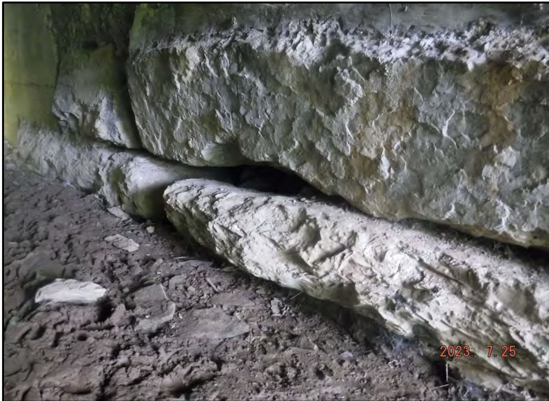
Photo 6: Typical Stone Masonry Abutment Open Joints
